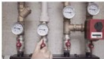
Smart Metering for Water and Electricity
